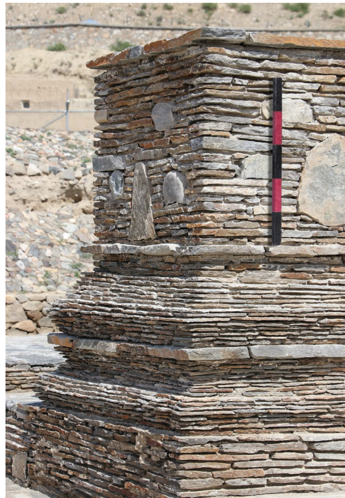
Detail of restored stone masonry on flanking wall of the south stair 2018
