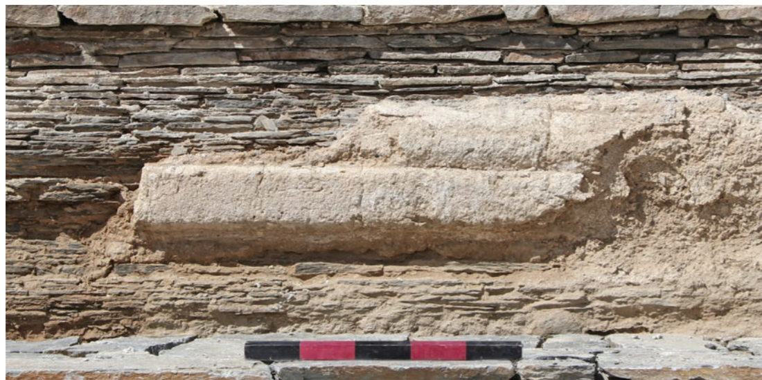
Detail of original lime plaster on west side of platform at Tepe Maranjan 2017
