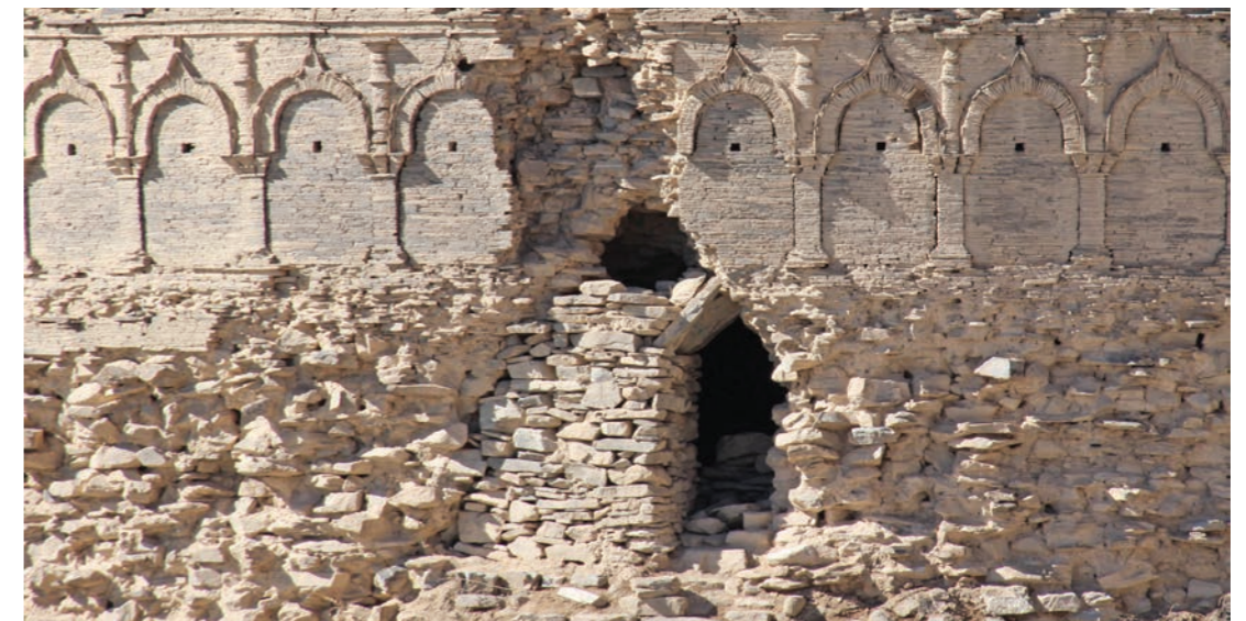
Cavity on east side of the lower drum of the stupa, before filling 2016
