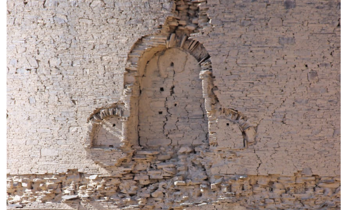
Upper niche on the east side of the stupa drum, prior to restoration 2016
